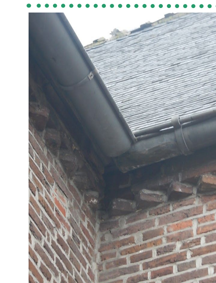
Lek in de dakgoten
