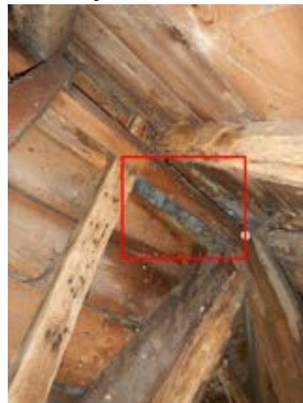
Dak [3]: ingerotte bebording.
