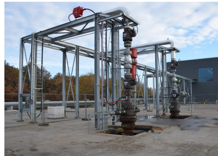
Diepe geothermie Mol
